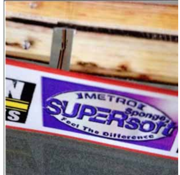
Figure 18 - Notch the lowermost bleacher.
